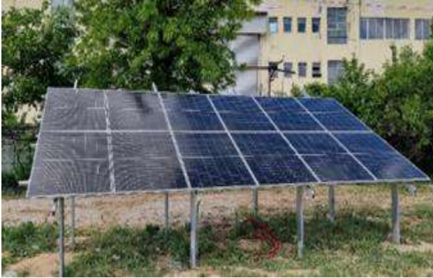
Fig. 1. Ground-mounted, bifacial photovoltaic panel system.
