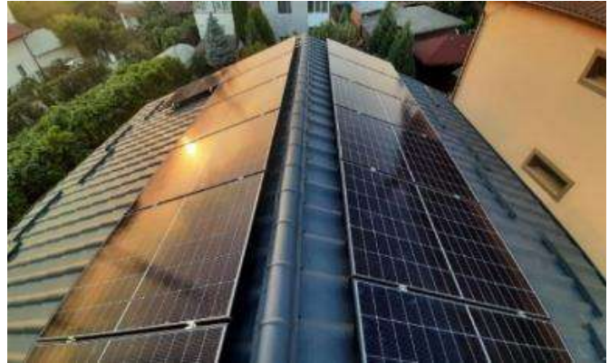
Fig. 2. Bifacial photovoltaic panel system installed on the rooftop of a residential building.
