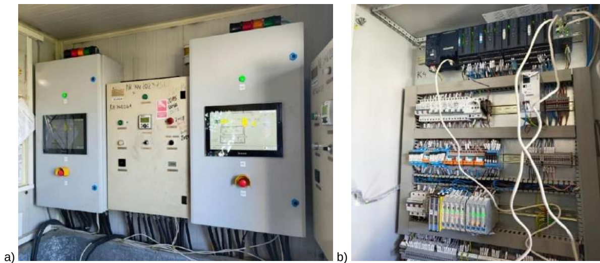
Fig. 2. a) The four automation cabinets; b) The interior of one of the automation cabinets (right)
