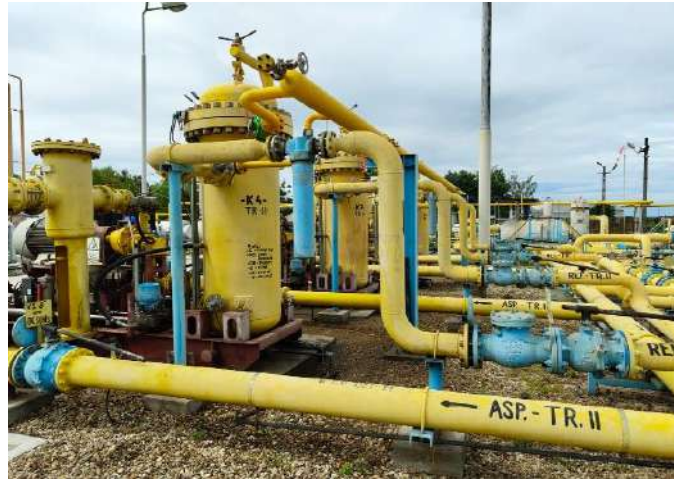
Fig. 1. The gas compressors located at Stoenești gas compression station
